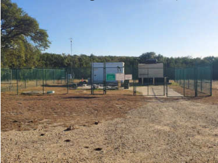
City of Killeen Sewage Lift Station
